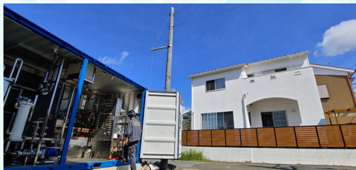
1st containerized plant for black water treatment and reuse in Japan
