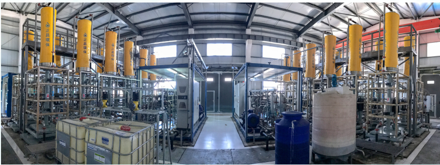
RO concentrate recovery
